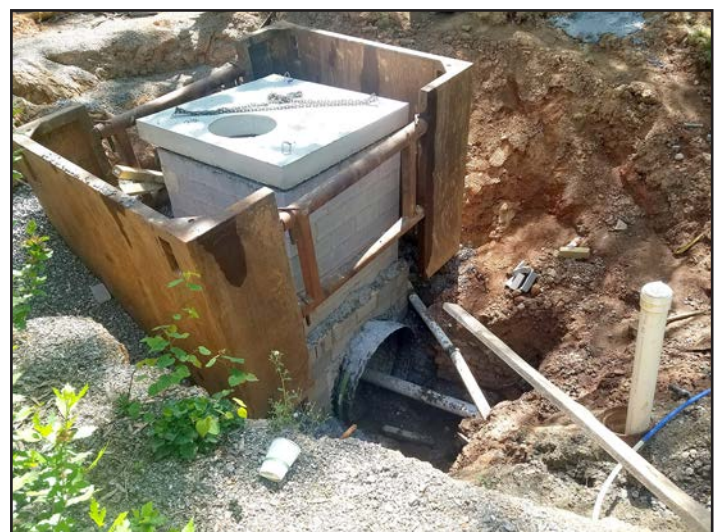
Some progress is being made with the Montford Avenue sinkhole. All concerned are looking forward to the system connections being completed. Stay tuned.
