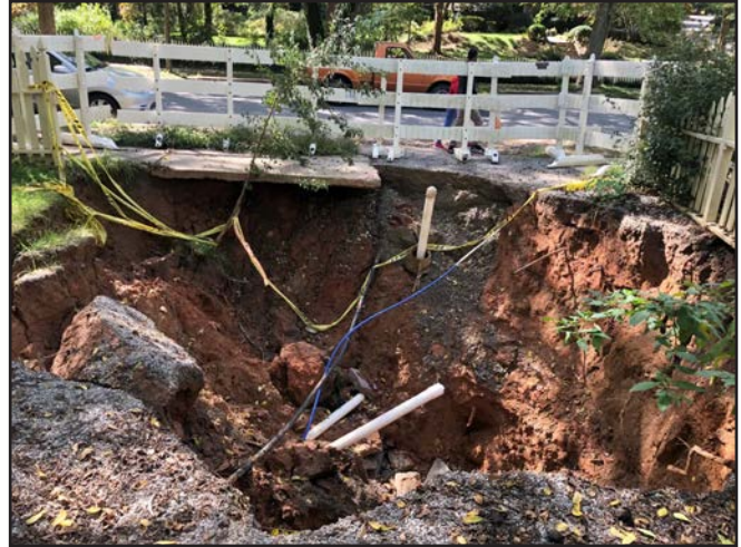
Pedestrians walk around the sinkhole on Montford Avenue in October. The problem started in July but got worse with torrential rains in August and September.
